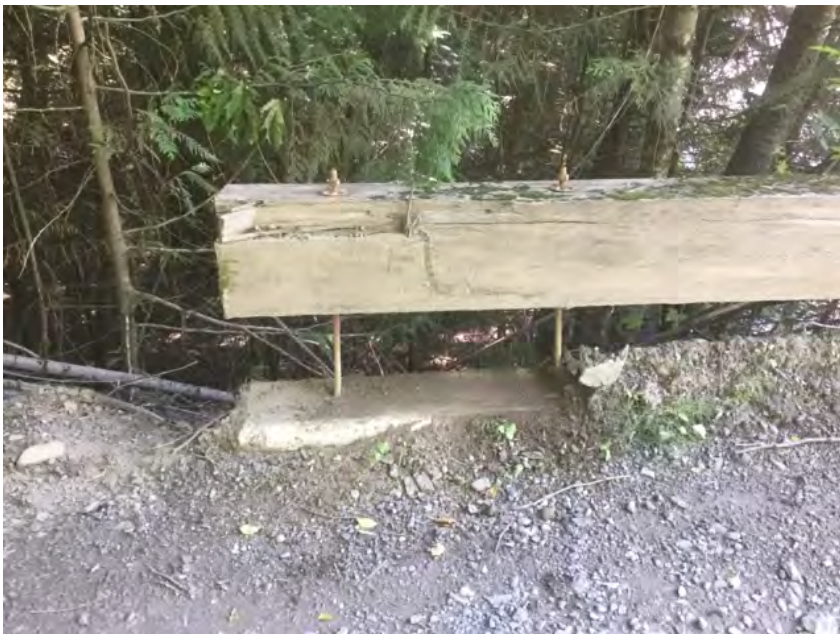
Missing riser at upstream right approach
